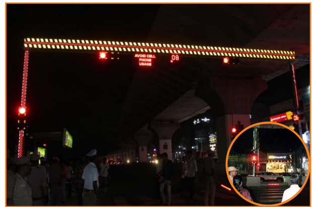
PELICAN SIGNAL (PEDESTRIAN CROSSING)
